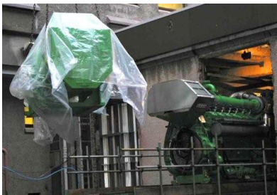
A CHP facility at the University
